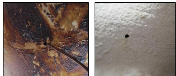
Figure 3. Hole in the Pipeline
